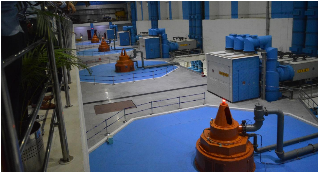
Four Hydro Power Units of 200MW
